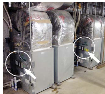
Steril-Aire UVC installation on heat pumps serving patient rooms at MCH
