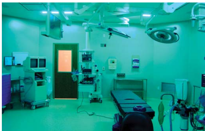
Custom-designed, ceiling-mounted UVC devices from Steril-Aire installed in Muskogee Community Hospital's surgical and procedural suites enable “after-hours” disinfection.
